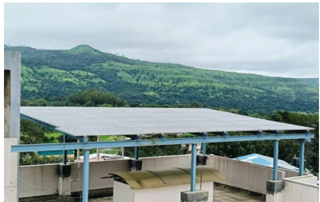
Solar panels ensuring uninterrupted education for girls in the Velhe hostel
