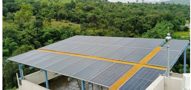
Solar panels installed at the girls' hostel in Velhe
